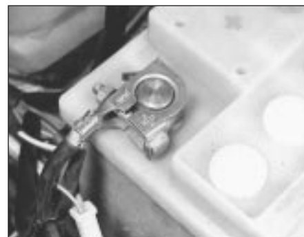
4.2 Battery positive terminal connection
