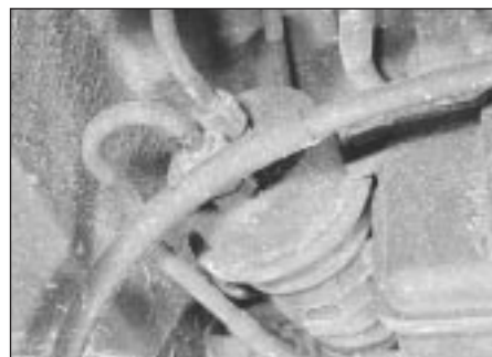
21.1 Fuel accumulator unit location
